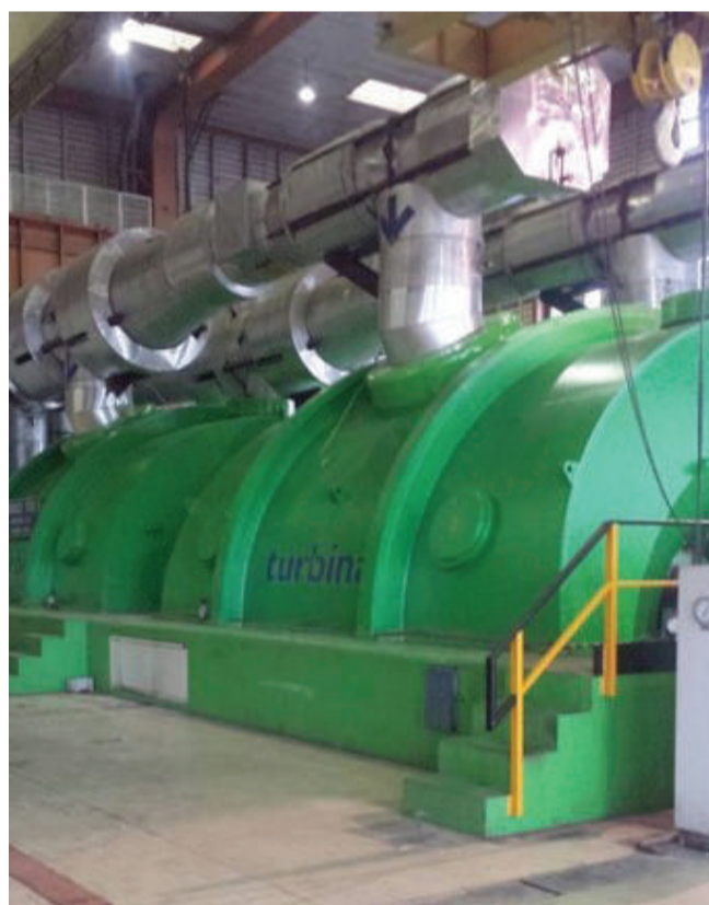
Franco Tosi steam turbine
