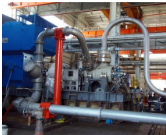
Main injection pump with electric motor, gearbox and suction & discharge piping
