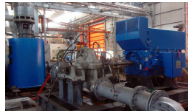
Test center auxiliary pump (left) and booster pump (center) with electric motor (right)
