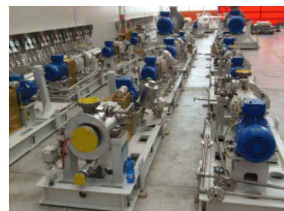
Area dedicated to process pumps
