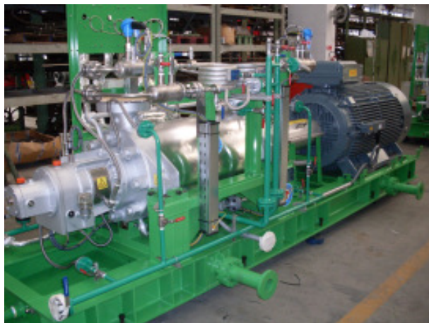
Boiler feed water pump
